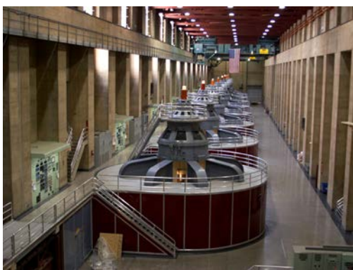
Figure 20.43 Hydroelectric generators at the Hoover dam. (credit: Jon Sullivan)
